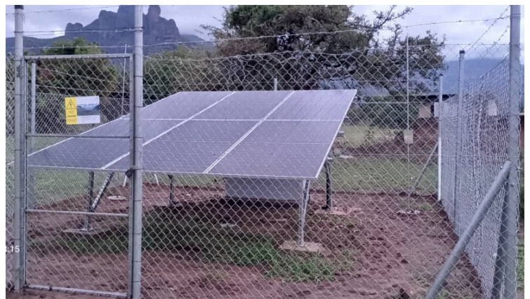
The 6 installed solar panels at Moruita HC2 through the advocacy efforts of women advocates
